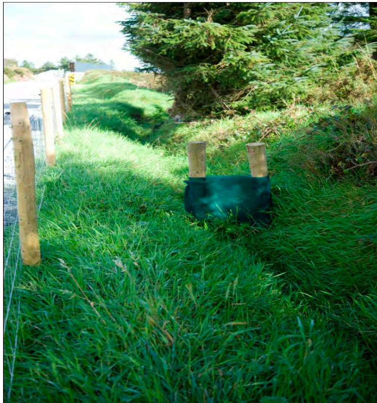
Figure 4: Silt Trap across Grassed Swale
